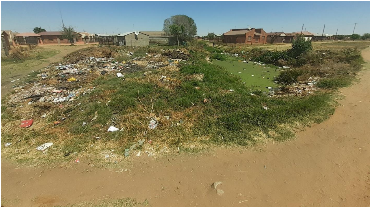
Figure 15: Illegal dumping in a storm water drainage (Nkoane road, Thabong)
